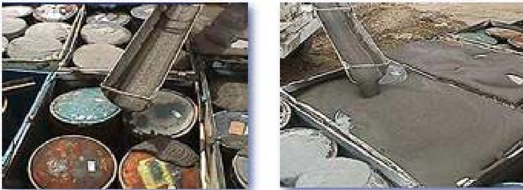
Figure G3-2. Filling voids around drums at EnergySolutions Facility in Utah. Figure taken from EnergySolutions Web site.
