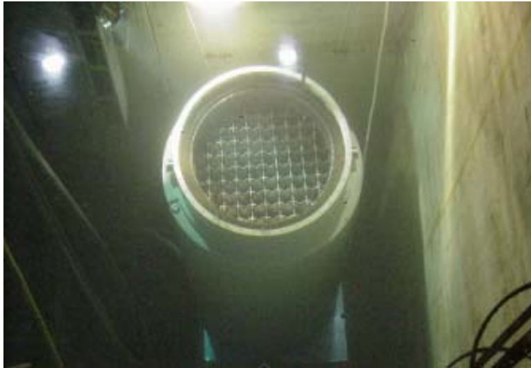
Figure G2-2. Holtec International cask in fuel storage pool). Figure taken from Holtec International Web site.
