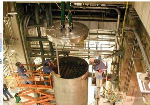
Fit up of the MPC and MPC Lid at J.A. FitzPatrick Nuclear Plant
