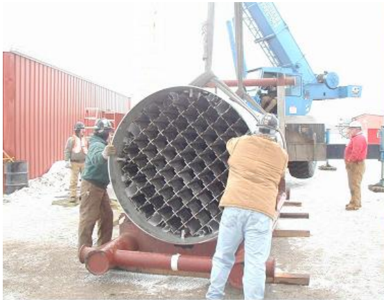
Receiving the MPC at J.A. FitzPatrick Nuclear Plant
