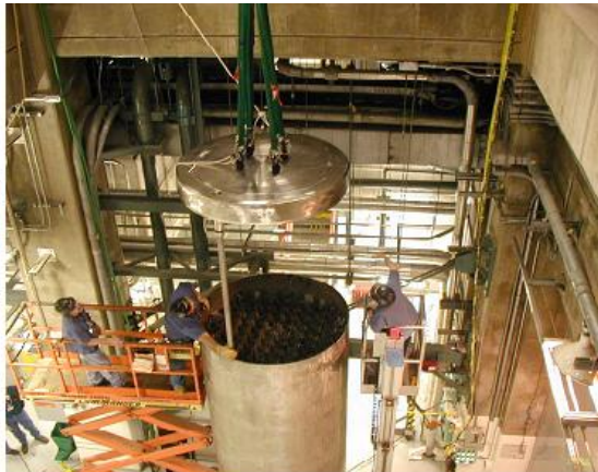
Fit up of the MPC and MPC Lid at J.A. FitzPatrick Nuclear Plant
