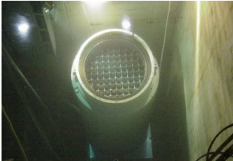
Figure G2-2. Holtec International cask in fuel storage pool). Figure taken from Holtec International Web site.
